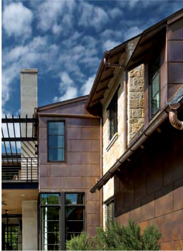
13 AN EXAMPLE OF WEATHERED COPPER SIDING
